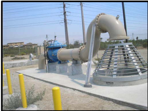
CB-20 Turnout Facility
