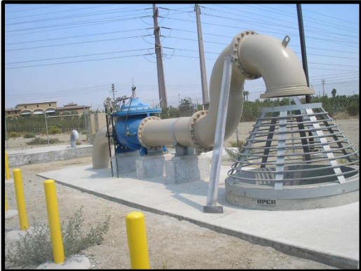
CB-20 Turnout Facility
