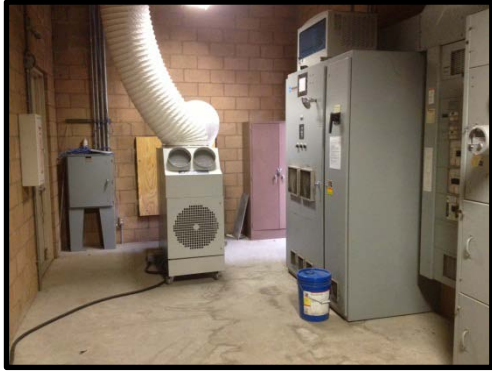
MCC Control Panel
