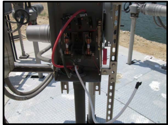
Damages to new electrical enclosure
