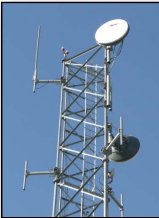
Basin Communication Tower
