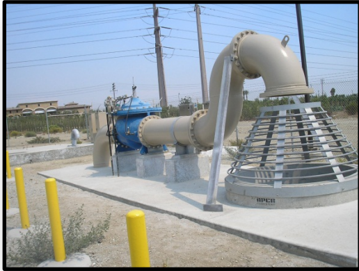
CB-20 Turnout Facility
