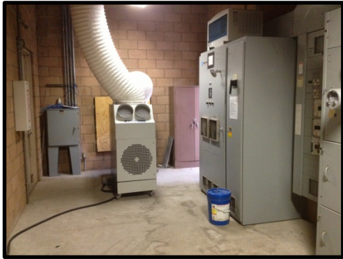
MCC Control Panel
