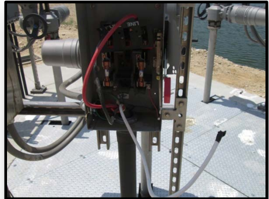
Damages to new electrical enclosure
