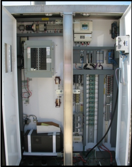
San Sevaine Turnout Control Panel
