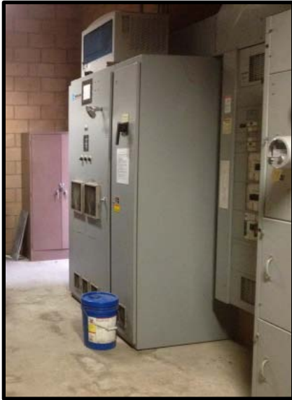
Existing MCC Control Panel
