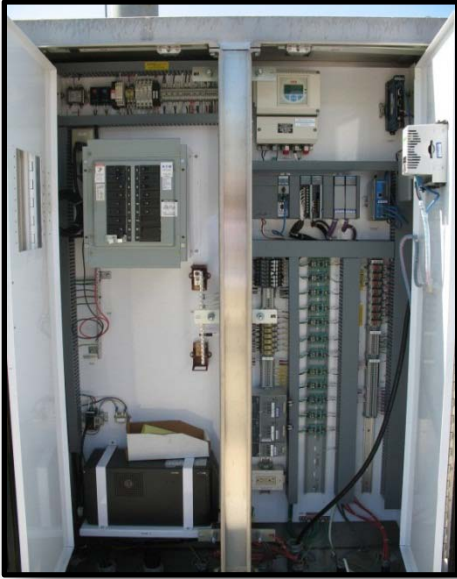
San Sevaine Turnout Control Panel
