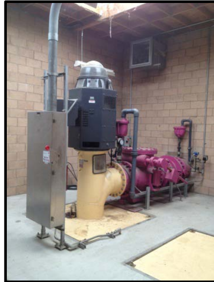
Existing Pumping System
