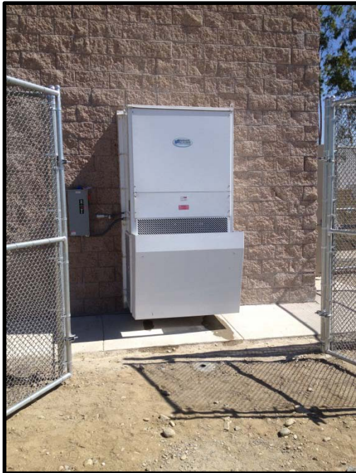
Installed AC Unit
