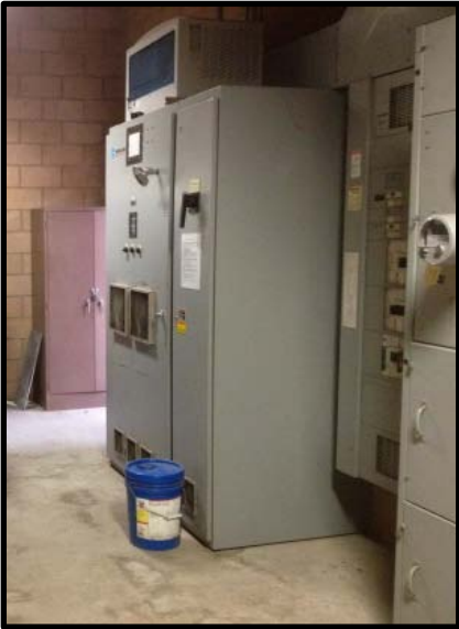
Existing MCC control panel
