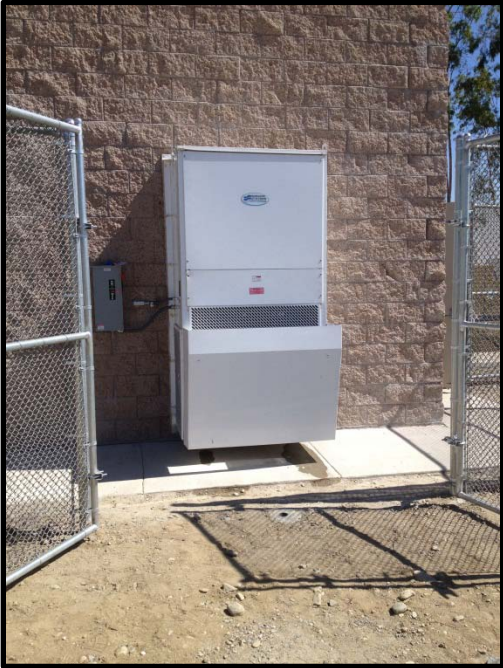
Installed AC unit
