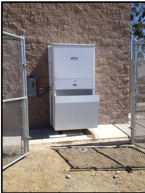
Installed AC unit
