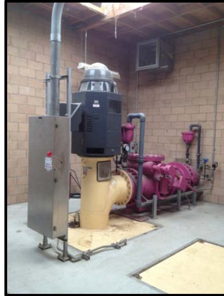
Existing pumping system
