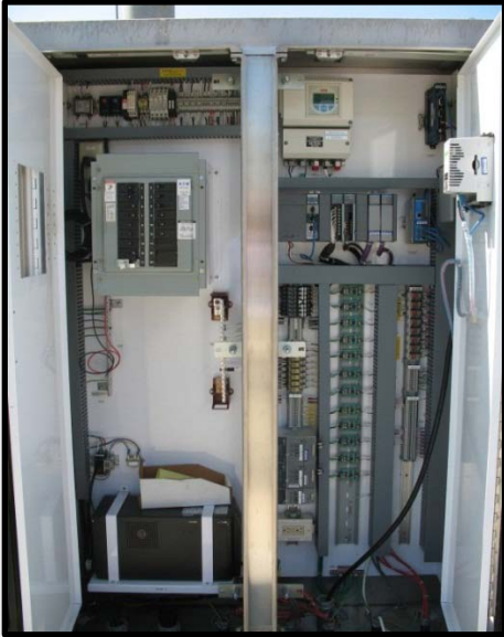
San Sevaine turnout control panel
