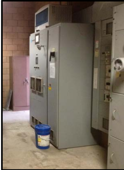
Existing MCC control panel
