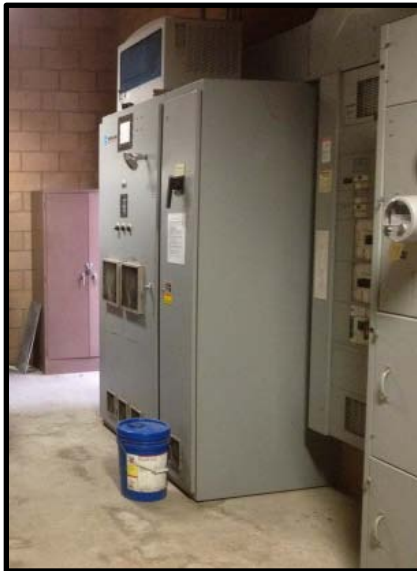
Existing MCC control panel
