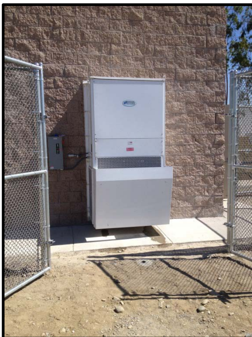
Installed AC unit
