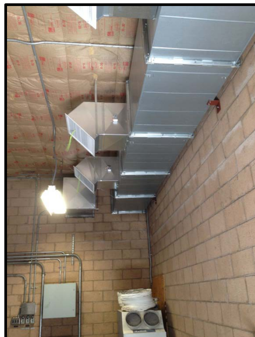
Installed ceiling insulation and AC air ducting
