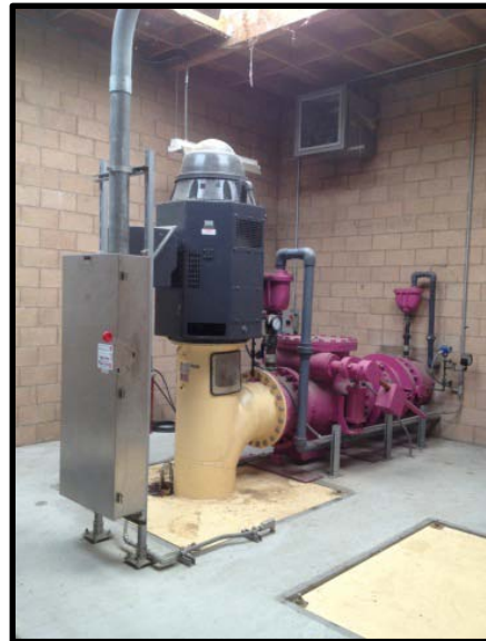
Existing pumping system
