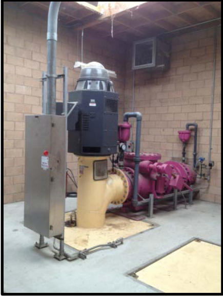
Existing pumping system
