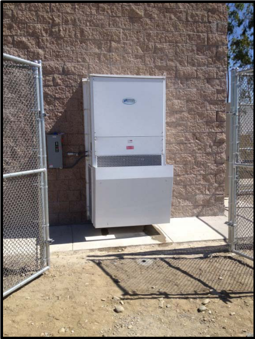
Installed AC unit
