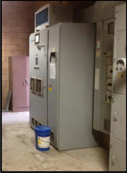
Existing MCC control panel
