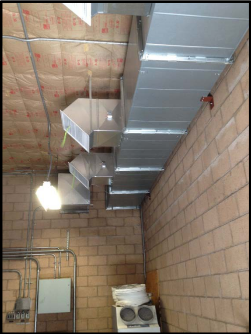
Installed ceiling insulation and AC air ducting
