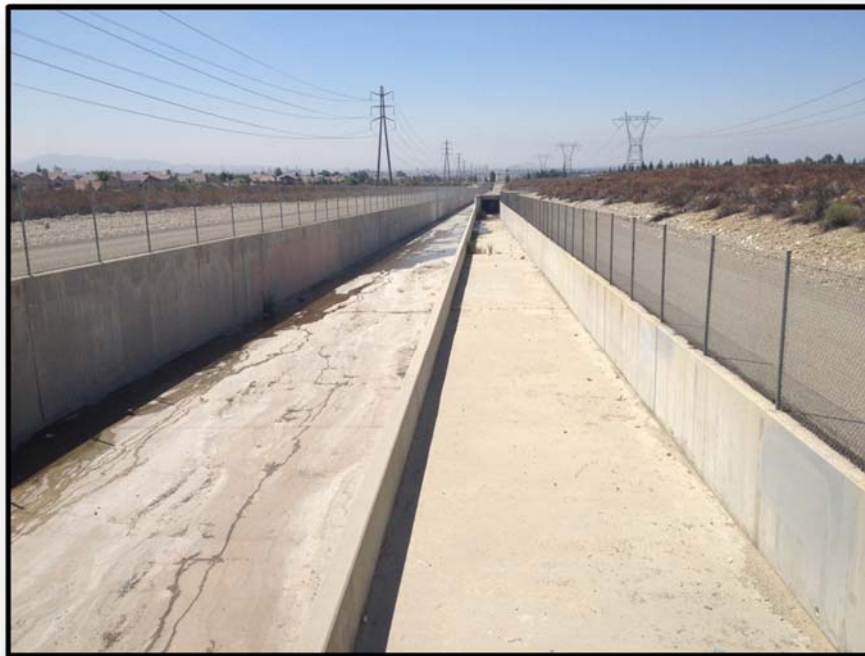
Field photo showing the location of the proposed improvement to the existing channel to increase storm water capture
