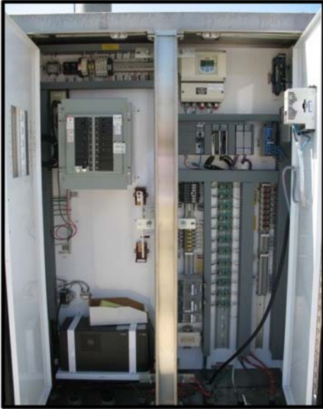
San Sevaine turnout control panel
