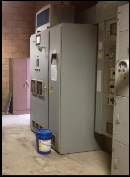
Existing MCC control panel
