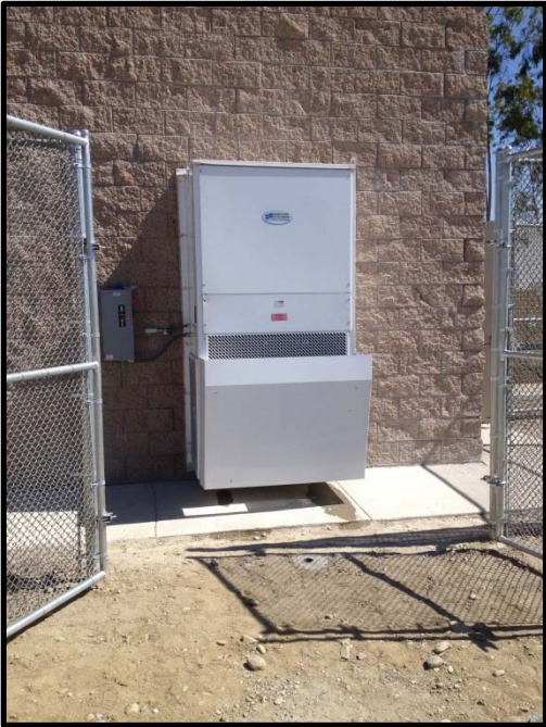
Installed AC unit
