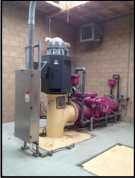
Existing pumping system
