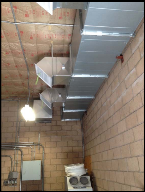
Installed ceiling insulation and AC air ducting
