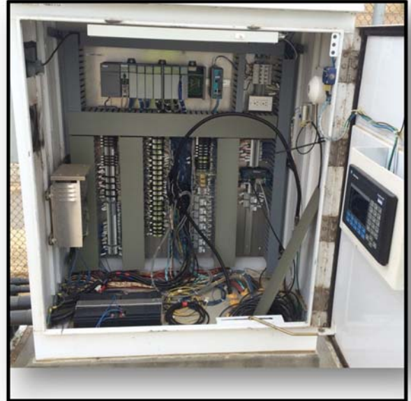
Turner Basin control panel
