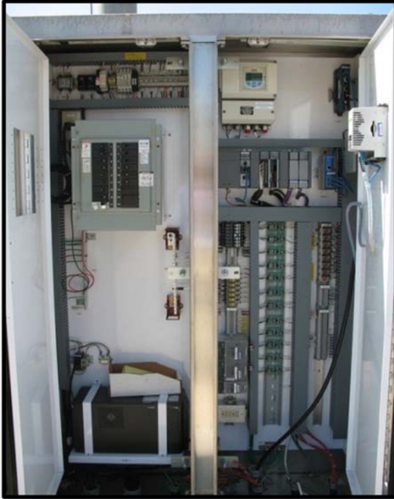
San Sevaine Turnout control panel
