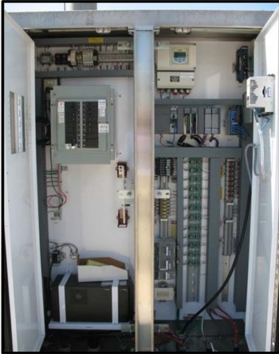
San Sevaine Turnout control panel
