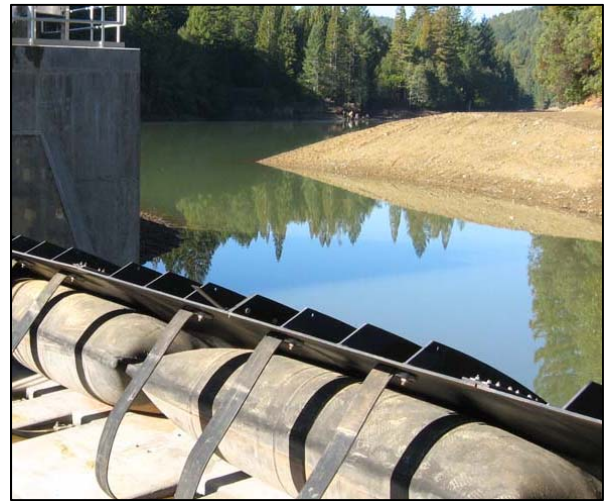
An Obermeyer Weir Wall example in Mendocino, California
