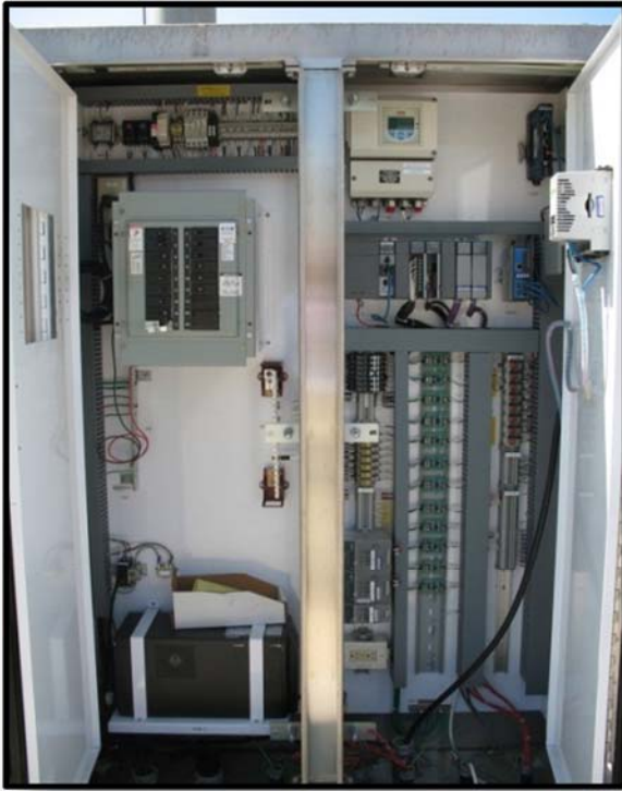
San Sevaine Turnout control panel
