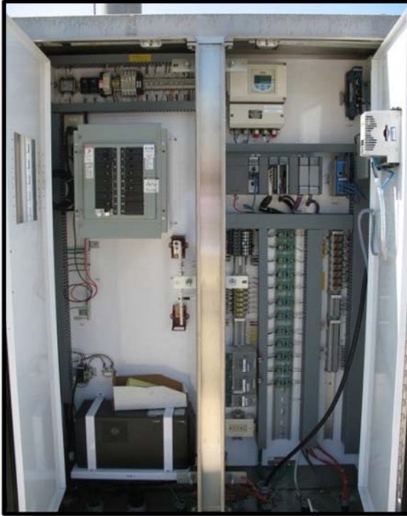
San Sevaine Turnout control panel
