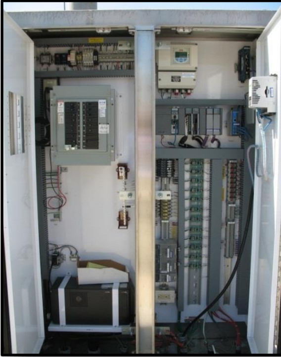
San Sevaine Turnout control panel
