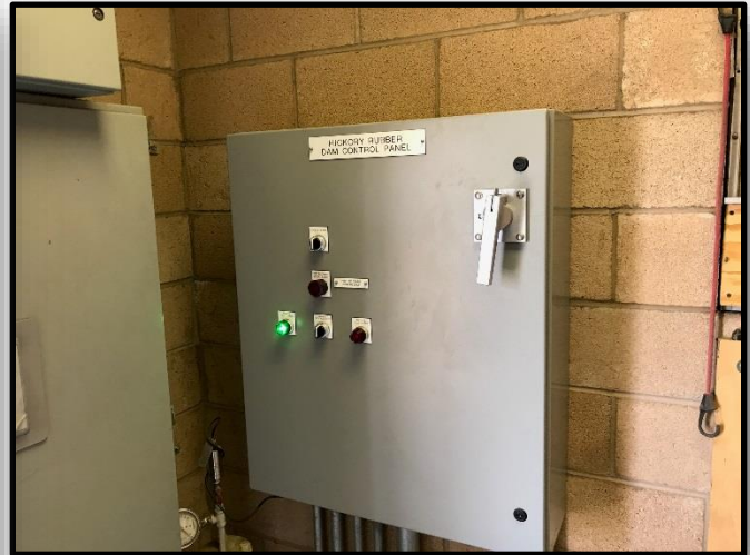
Rubber Dam control panel
