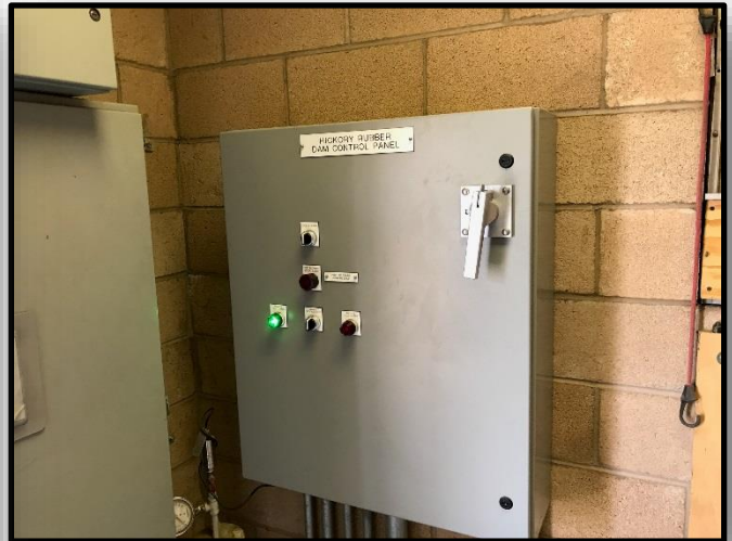
Rubber Dam control panel
