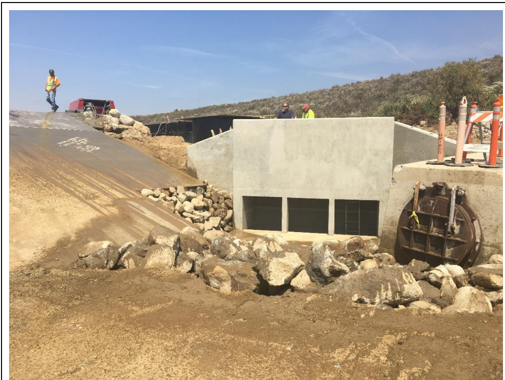
Storm water inlet structure additional view
