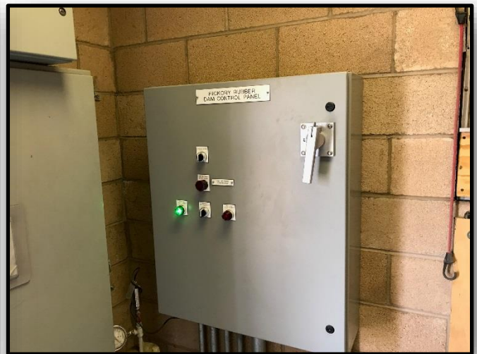
Rubber Dam control panel
