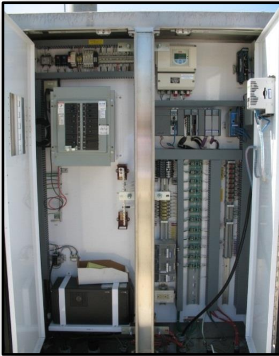
San Sevaine Turnout control panel
