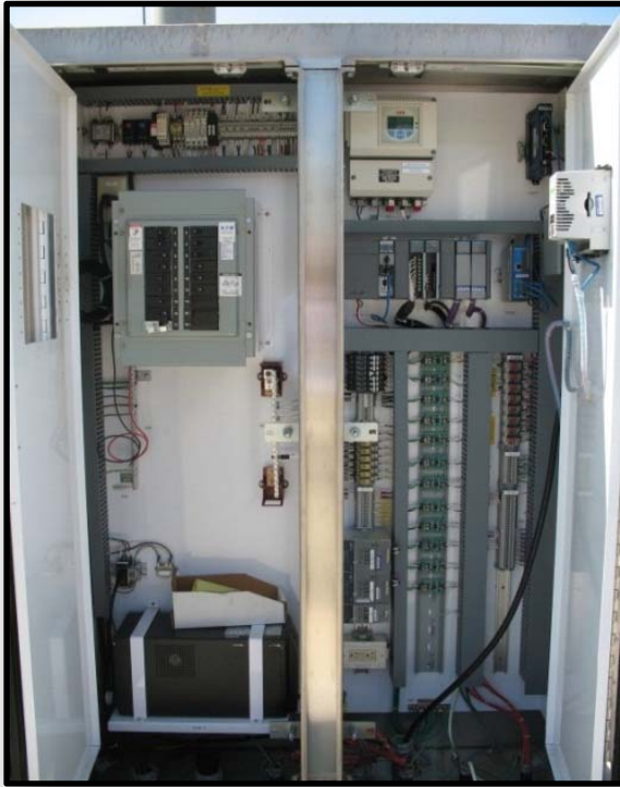
San Sevaine Turnout control panel
