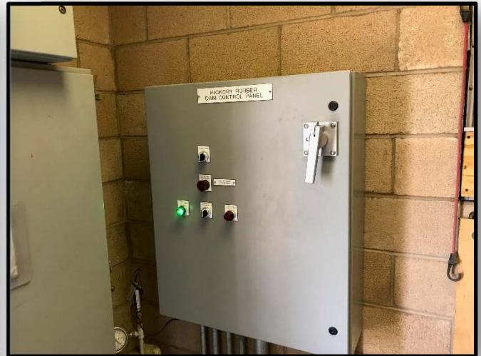
Rubber Dam control panel
