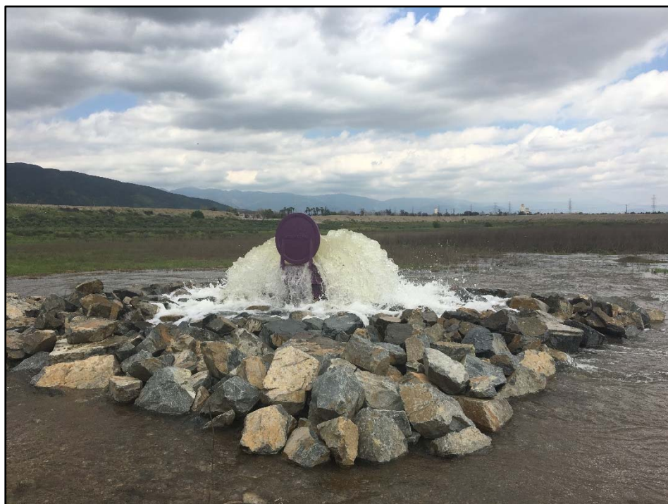
Full operation of pump system - Outlet Structure in Basin 2
