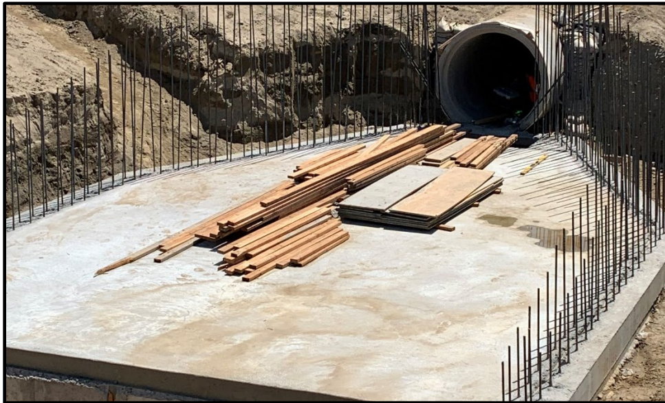
Wineville/Jurupa Storm Water Distribution Pipeline (Construction of the Inlet Structure for the Forebay in Wineville Basin)
