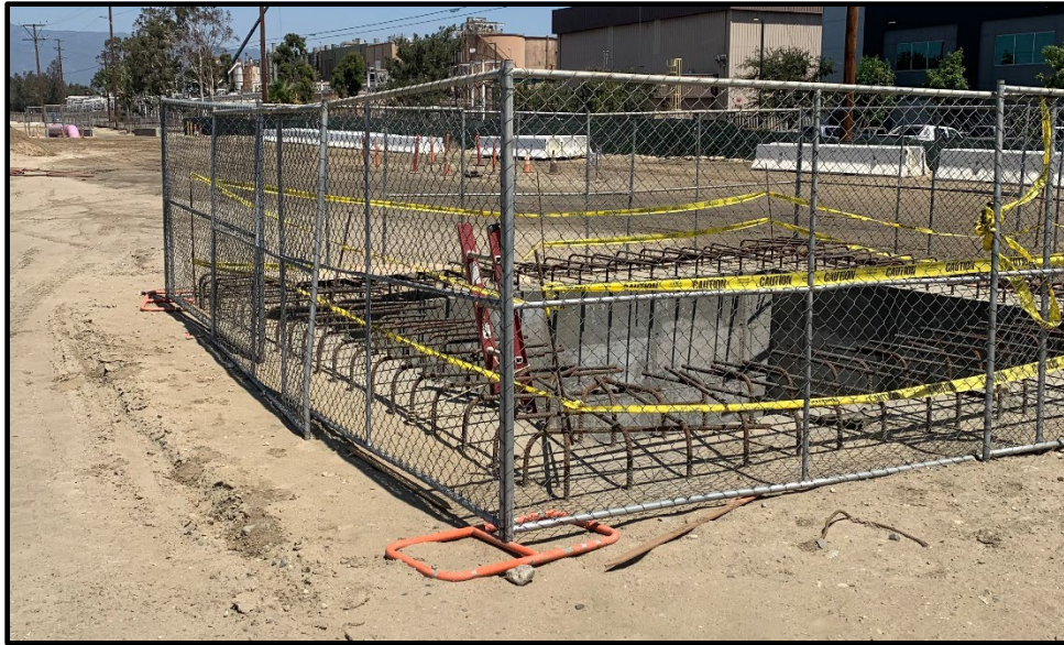
Wineville/Jurupa Storm Water Distribution Pipeline (Wet Well Construction Reaching Top of Grade)
