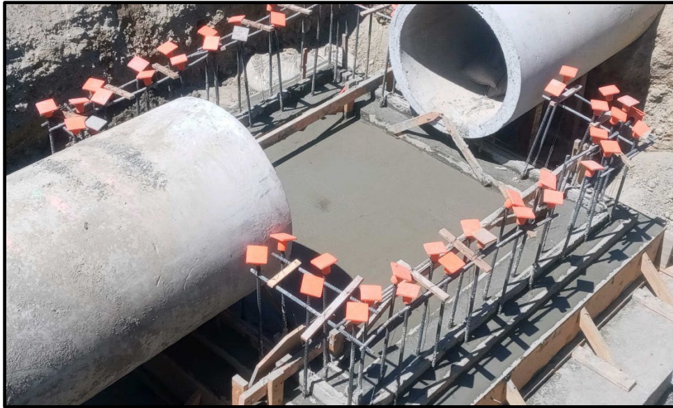
RP3 Basin Improvement (Construction of Foundation for the Diversion Structure at RP3)
