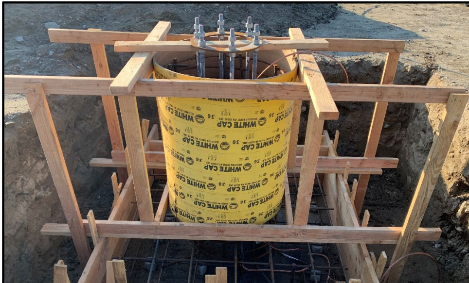
Wineville/Jurupa Storm Water Distribution Pipeline (Construction of the Monopole Foundation at Wineville)
