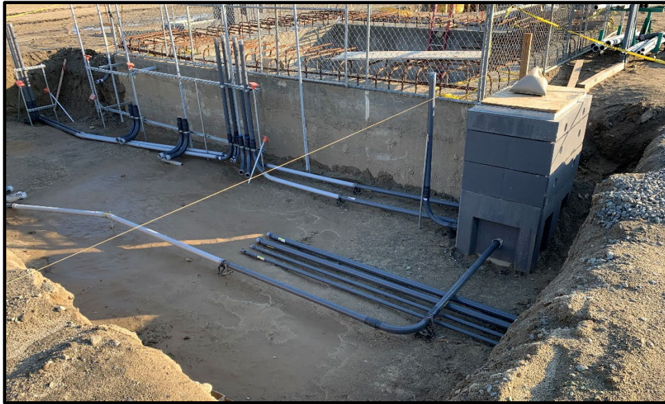
Wineville/Jurupa Storm Water Distribution Pipeline (Wet Well Construction Preparation of Slab with Underground Conduit)
