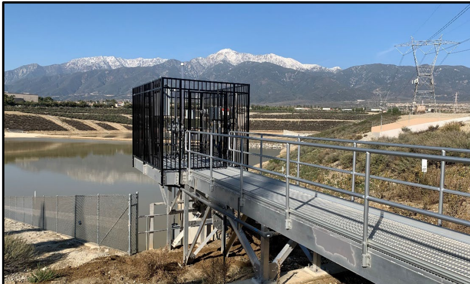
Lower Day Basin Improvement (Completed Catwalk Platform for new gates and level sensors at Cell 3)
