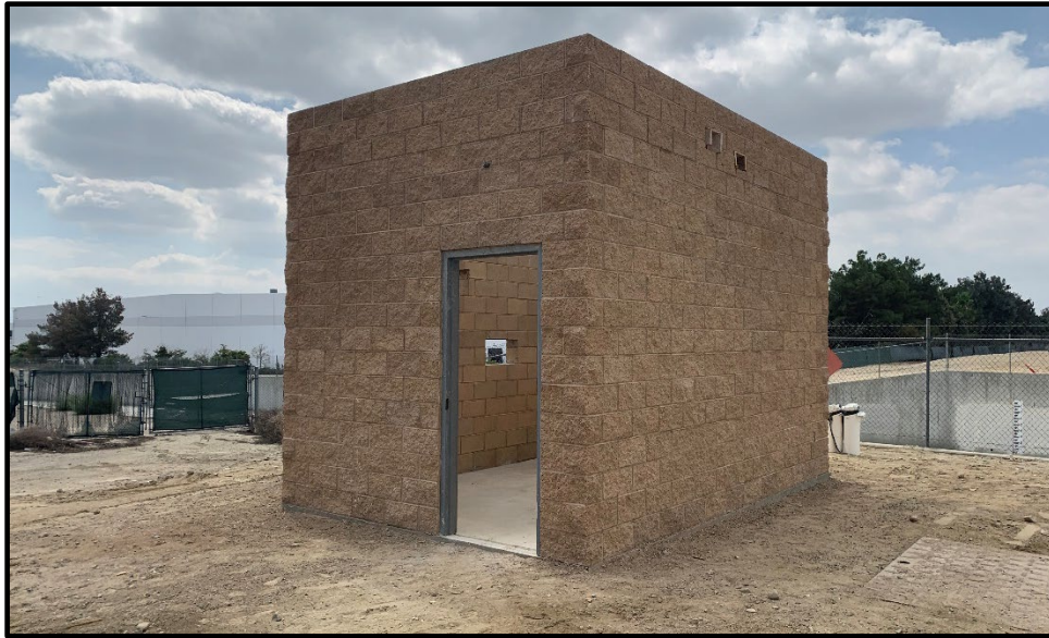
Wineville Basin – Rubber Dam Control Building (Completed CMU Wall – Pending Roofing Materials)
