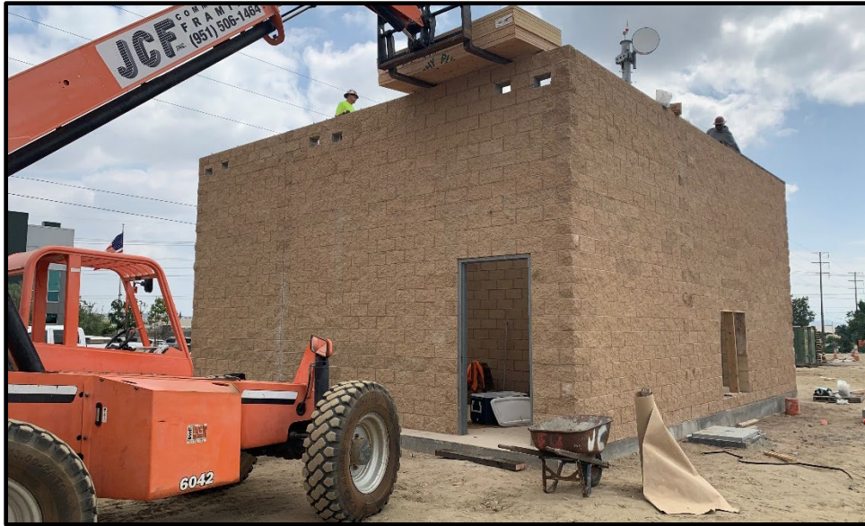
Wineville Basin – Pump Station Building North Side (Completed Wall – Joist Beam Installation)
