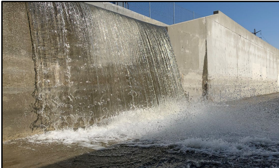
Lower Day Basin Improvement – Day Creek Diversion (Test Operation of Gate Dam System – Onto Diversion Channel)
