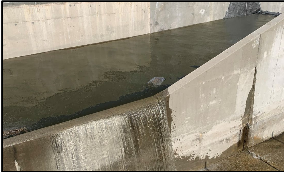
Lower Day Basin Improvement – Day Creek Diversion (Test Operation of the Gate Dam System – Main Channel)
