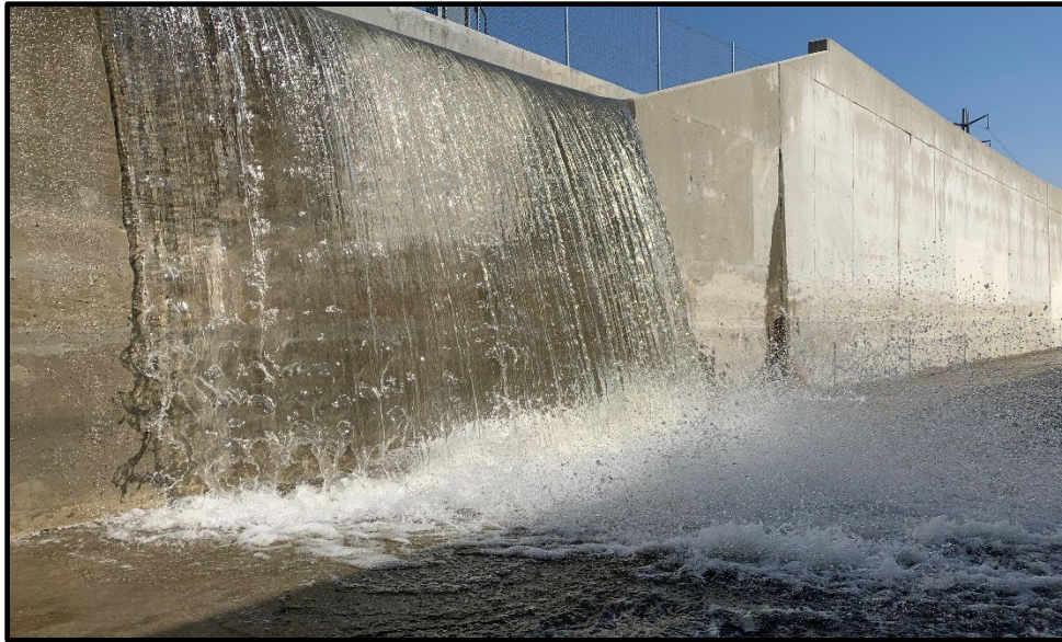
Lower Day Basin Improvement – Day Creek Diversion (Test Operation of Gate Dam System – Onto Diversion Channel)
