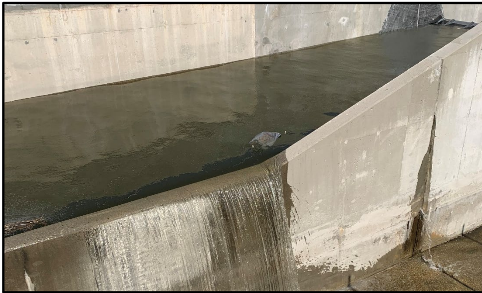
Lower Day Basin Improvement – Day Creek Diversion (Test Operation of the Gate Dam System – Main Channel)
