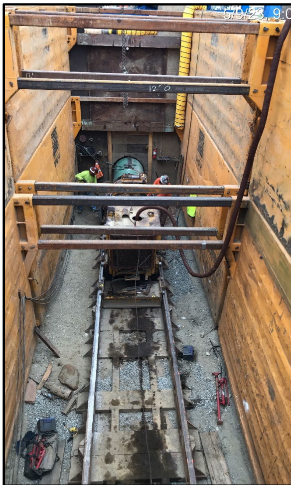
Wineville/Jurupa Storm Water Distribution Pipeline (Jacking Pit for the Boring Operations at Jurupa Road/Street)
