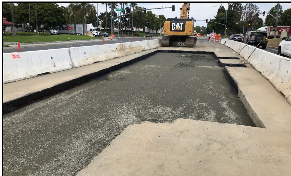
Wineville/Jurupa Storm Water Distribution Pipeline (Asphalt work at Jurupa Road/Street for the New 30-inch Pipeline)
