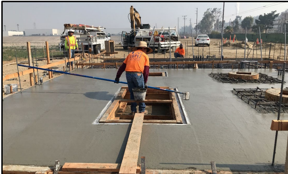
Wineville/Jurupa Storm Water Distribution Pipeline (Construction Slab Floor for New Pump Station at Wineville)
