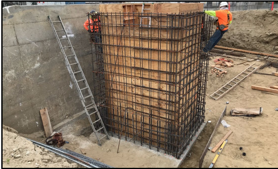
Wineville/Jurupa Storm Water Distribution Pipeline (Gate Structure Pit for Wineville Basin Outlet Gate System)
