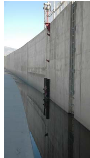
New inlet gate in San Sevaine Channel to Jurupa Basin
