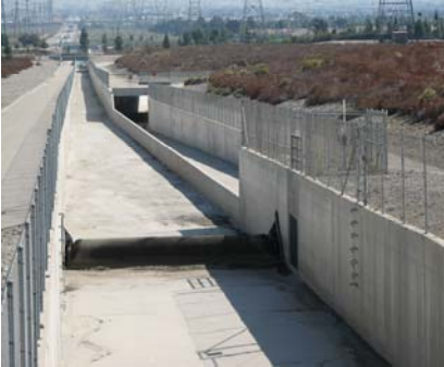
Rubber dam inflated near Lower Day Basin
