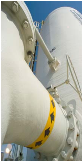
Desalter Product Water Tank
