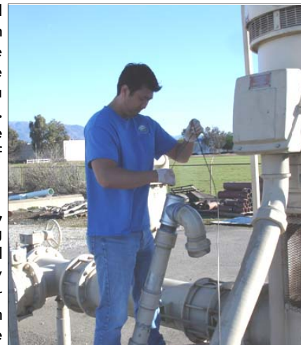
Installing a pressure transducer
